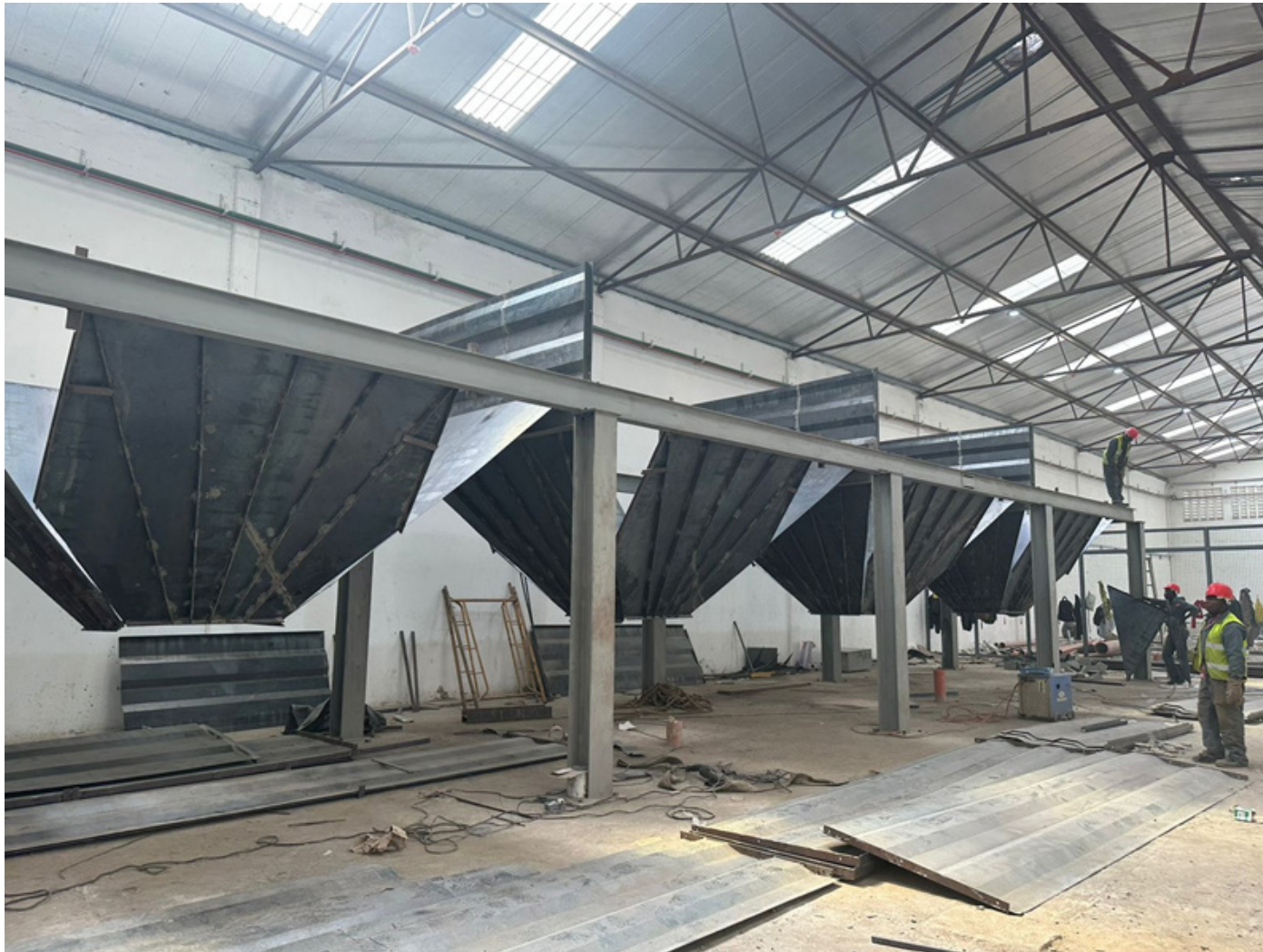
Grain silos being installed at the mega kitchen that can hold up to 40 tons of grains each.
